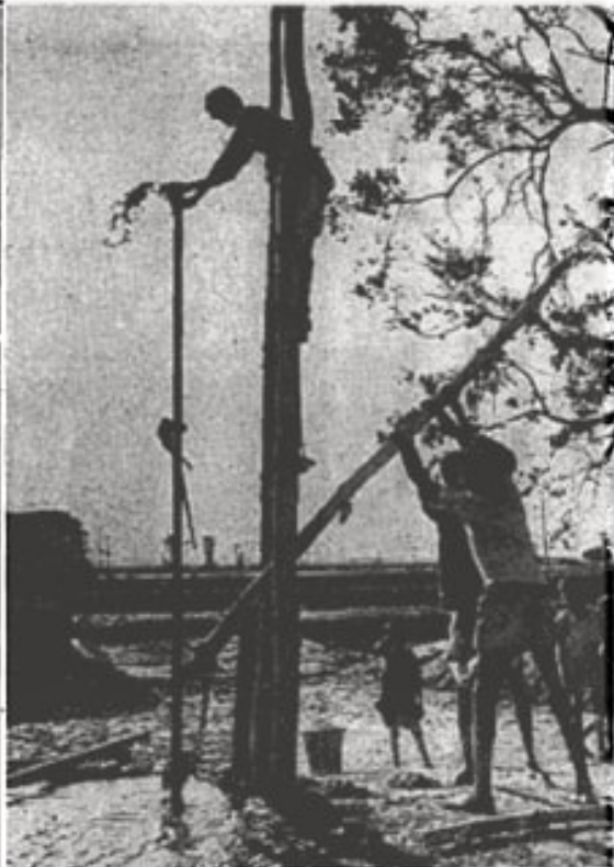
Villagers in the Gaya district of Bihar dig for water. They force a pipe into the ground, then put another pipe through the first one and drive both deeper until they reach water. The entire operation may take one month.
